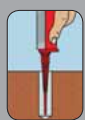
Fill with composite mortar starting from drill hole base (see enclosed leaflet)
