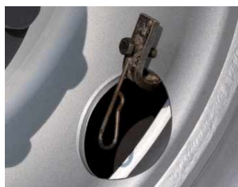
Missing hose valve extension
