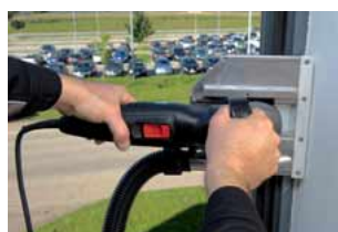
Old windows are separated from the reveal with a single cut and almost no dust. Fast, precise and requires very little expenditure of force.
