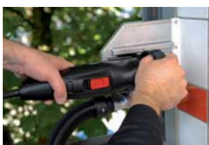
The large diamond cutoff wheel effortlessly separates tiles, plaster and metal anchors.
