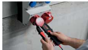
Voltage test with CEE socket
